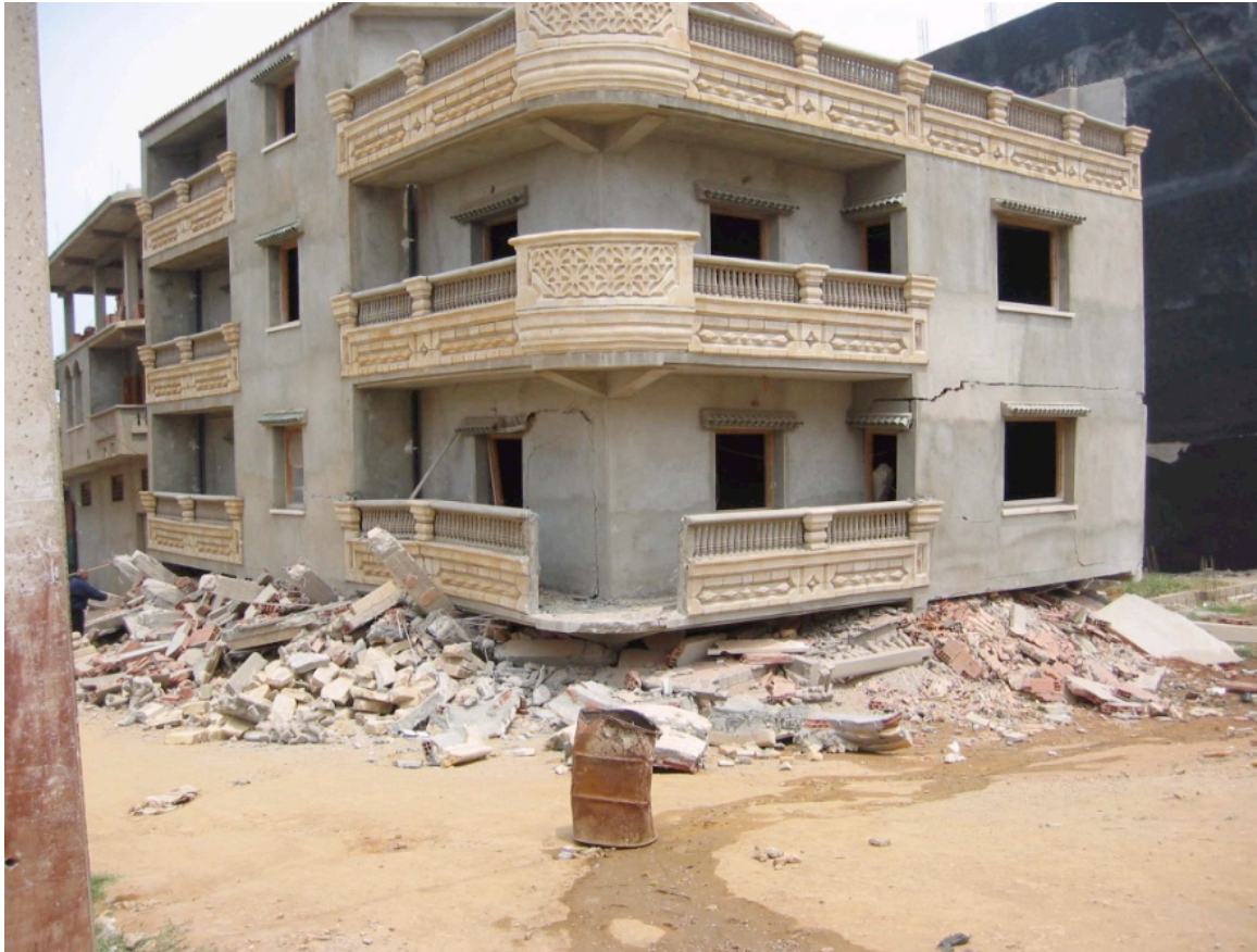
Vertical load collapse
